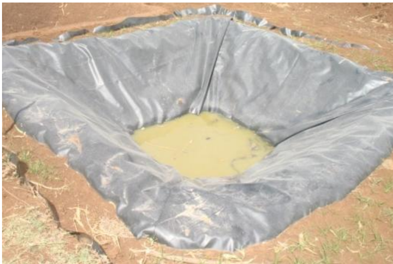
Figure 9. Geo-membrane lined pond
